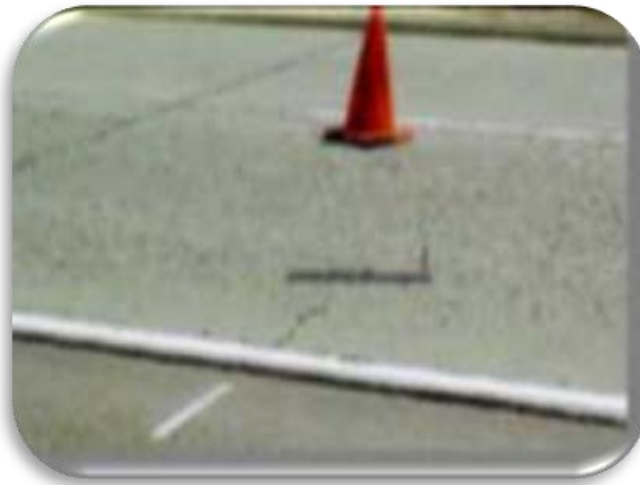
Figura N°3, fisura transversal o diagonal
