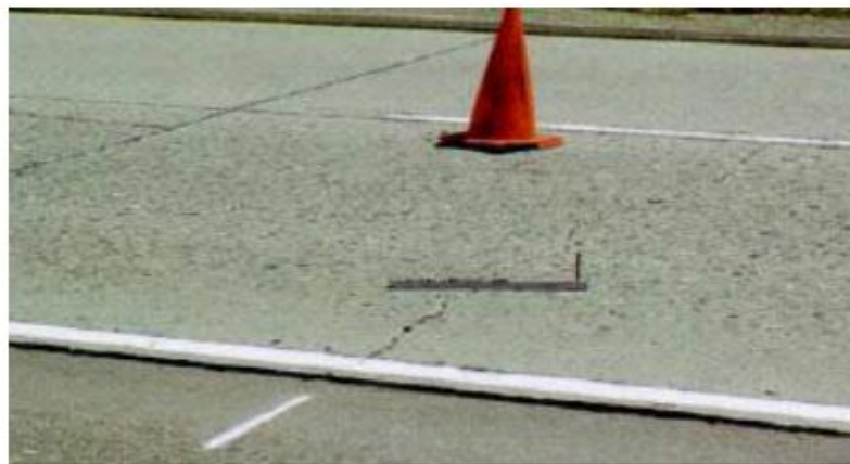
Fig. 3-15 FISURA TRANSVERSAL O DIAGONAL
