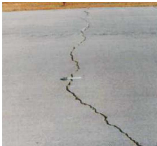
Figura 2.24 Fisura transversal o diagonal
