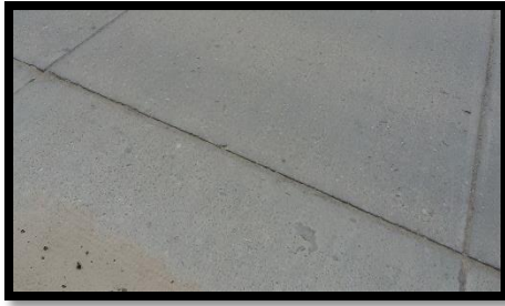
UM-13 (Prog. 0+596,433 a Prog. 0+621,690) Desnivel carril / berma
