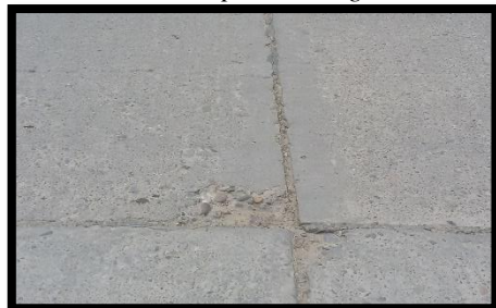
UM-16 (Prog. 0+731,310 a Prog. 0+757,388) Blow up / Buckling
