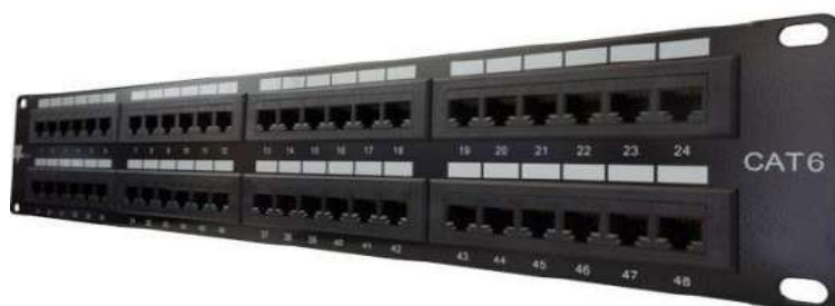
Figura 28. Patch panel 48 puertos
