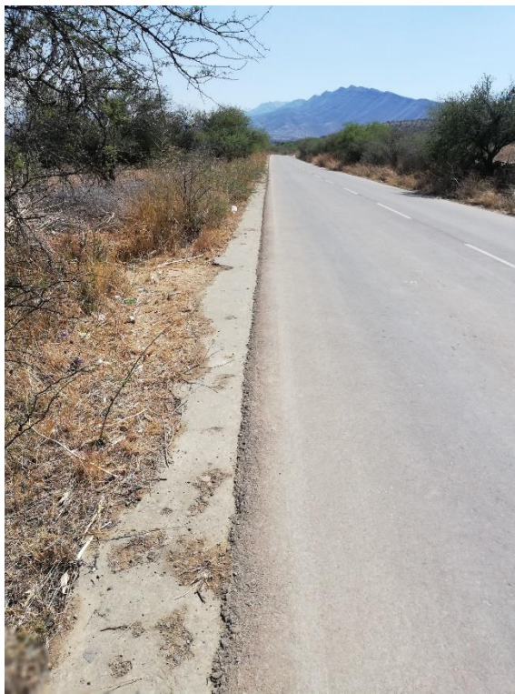
Desnivel carril berma
