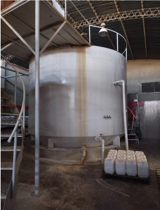
Figura 16 Reactor vista externa
