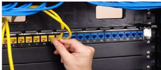
Figura 19. Patch panel ethernet
