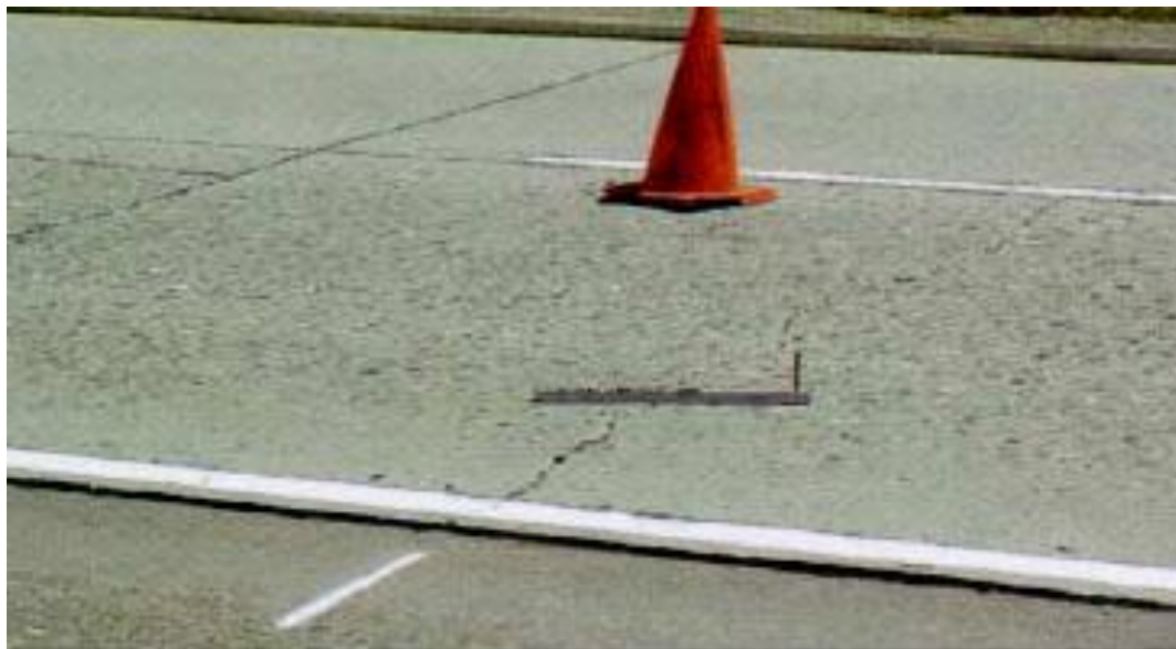
Fig.3.1. Fisura Transversal o Diagonal
